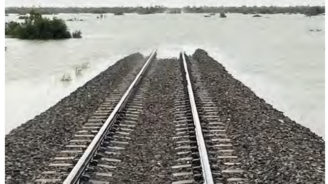
Rail access cut due to flooding in February 2024.
