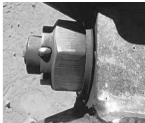
Figure 10: Mushrooming of the washer due to face wear into the bore.
